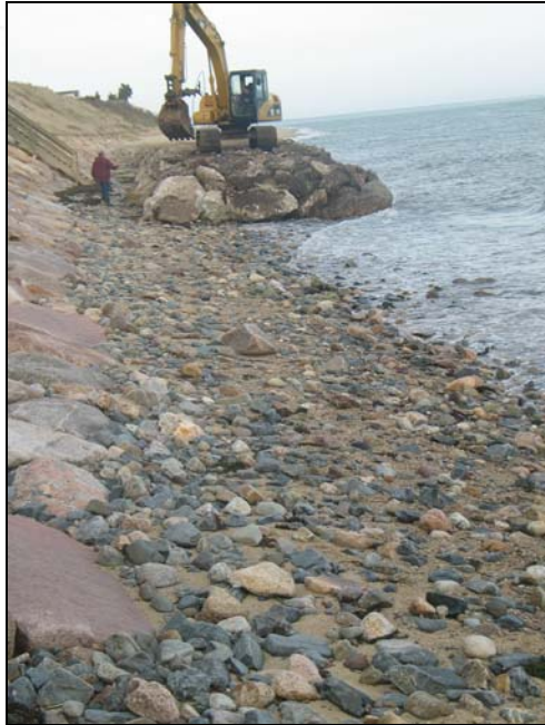
Figure 3. Photograph of the beach fronting 10 and 16 Triton Way during the access way installation.
